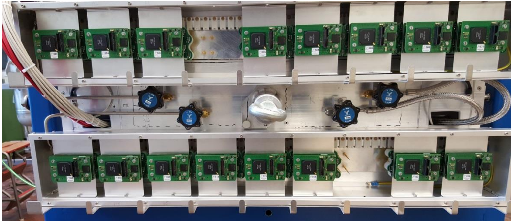
Read-out side with 16 stacked mezzanine cards.
