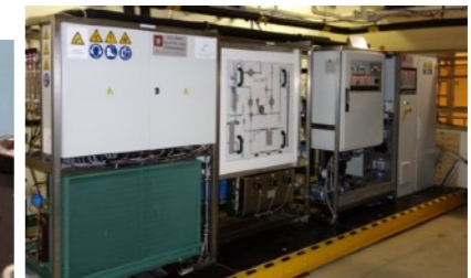
CO 2 cooling system
