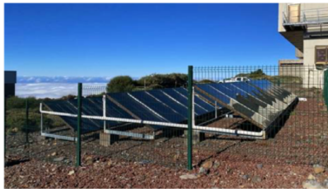
Solar Array: Ground-Mounted and Panel Canopy
