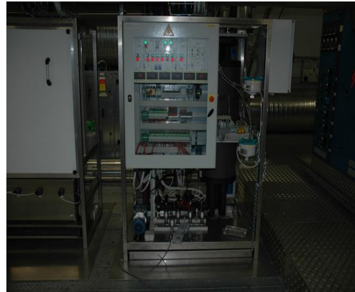
Server device for CO 2 cooling system
