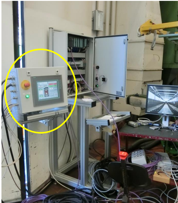
PLC controller for GERDA lock control in MPP
