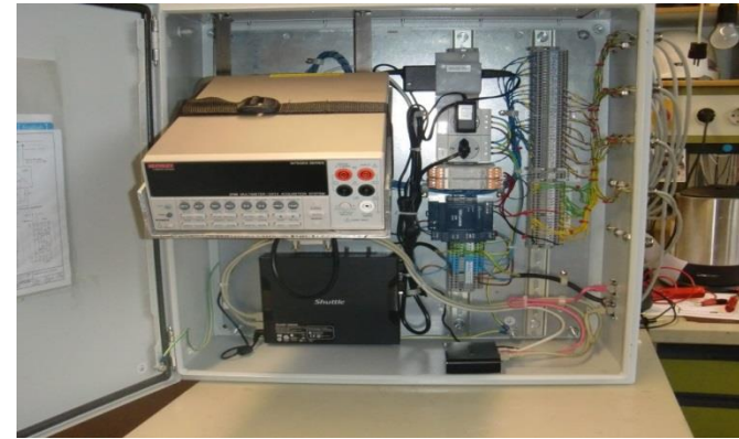
Remote pressure monitoring system
