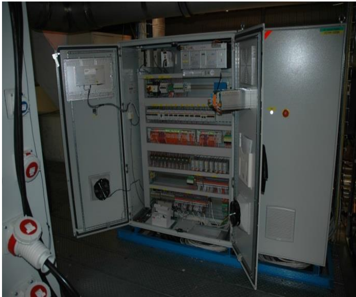
CO 2 cooling system at CERN
