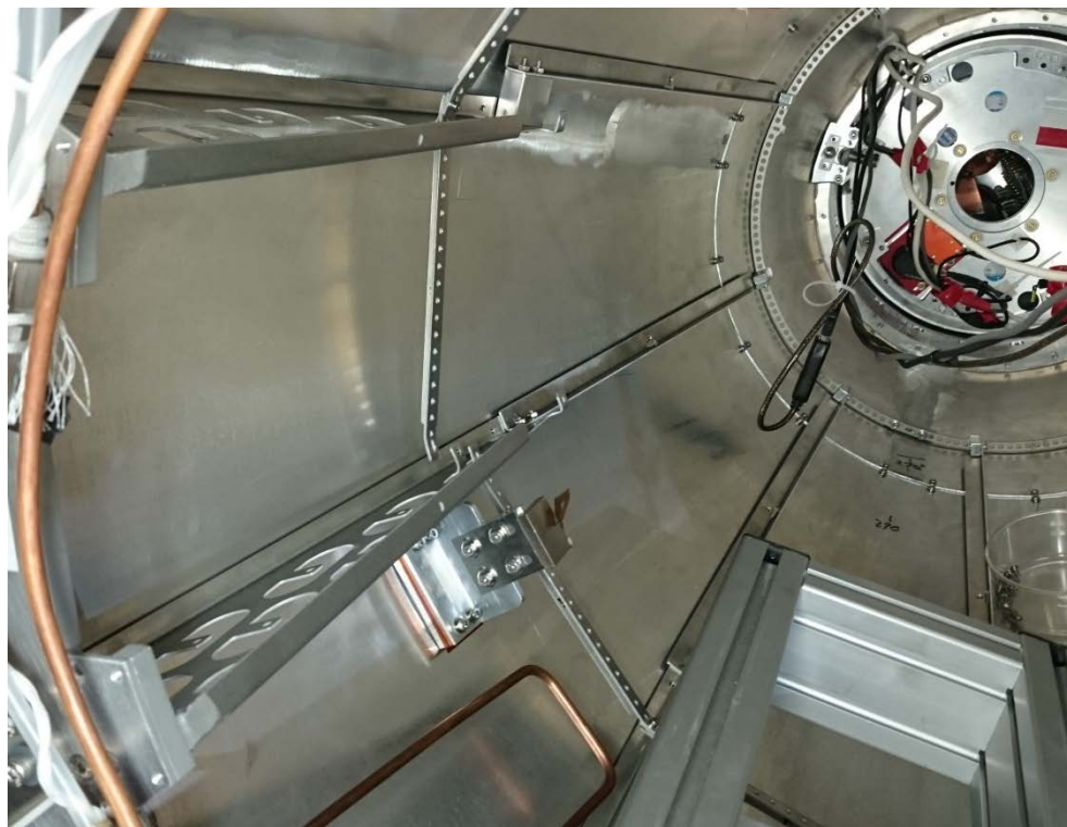
FWD CDC cable cage installed (inner spokes removed for B-Field Mapper installation)
