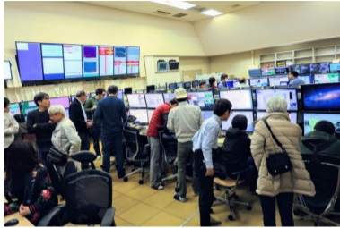
Control Room @ KEK, June 2019
