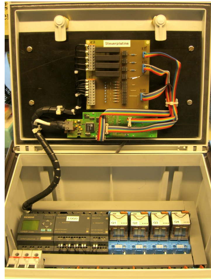
Shutter Control System
