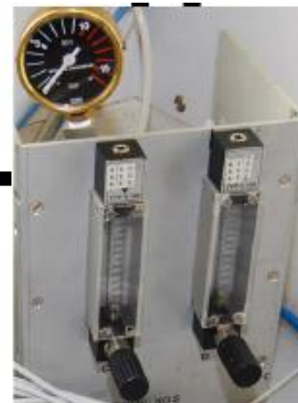
Manual flowmeters at outlet
