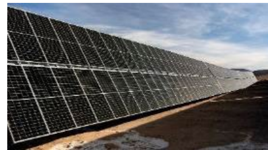
Power systems and eventual link to existing ESO PV plant
